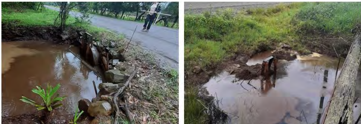
Figure 8-19: (Left) Floodgate ID 061G1 1.5 m culvert, invert level -1.2 m AHD, (Right) Floodgate ID 078G1 1.2 m diameter culvert, invert level -0.85 m AHD
