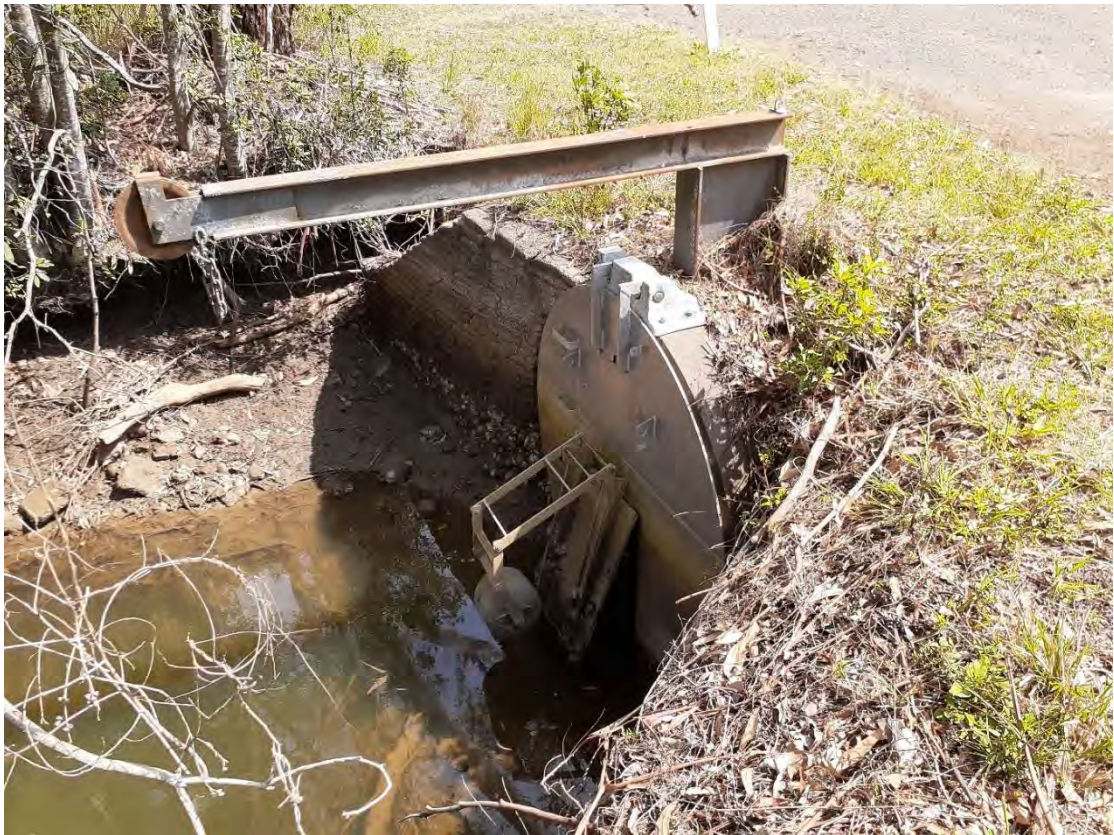
Figure 8-6: Example of an auto-tidal floodgate at FMS_26
