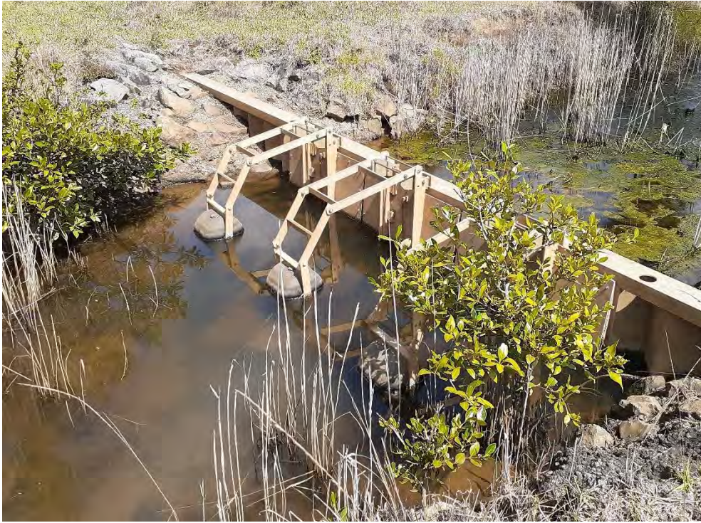
Figure 8-37: ID ASSS_61 - weir with auto-tidal gates
