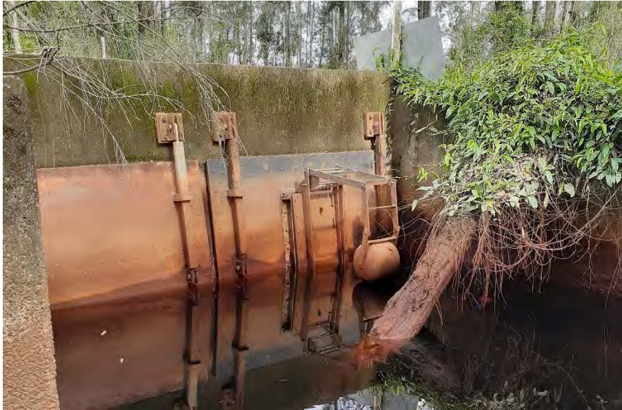
Figure 8-14: Floodgate ID 076G1 with auto-tidal buoyancy gate on the left bank floodgate
