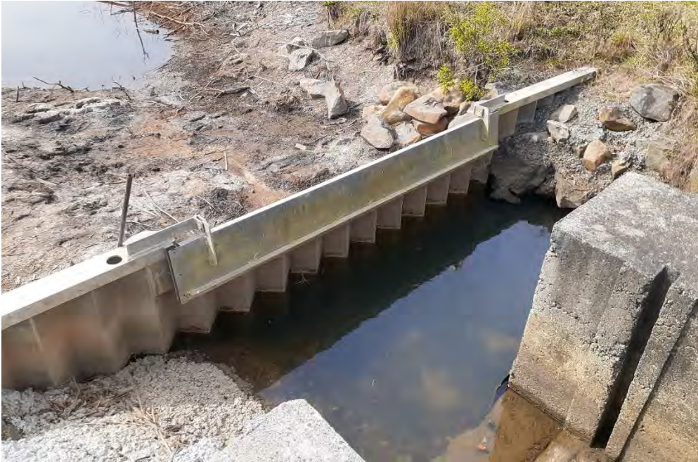
Figure 8-43: ID ASSS_45 floodgated weir with an invert of approximately 0.65 m AHD – note that upstream there is a dropboard weir structure downstream (with no boards in at the time of inspection)
