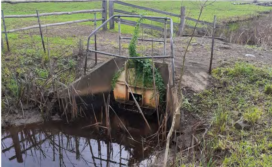
Figure 8-28: Floodgate ID 063G1 with sluice gate open
