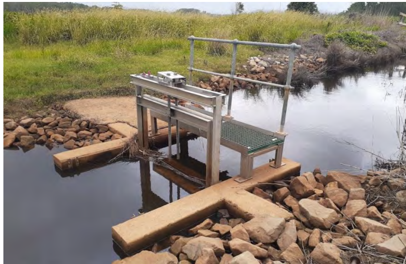
Figure 8-27: Water control structure F-2230-FH on Maloneys Drain (crest level ~0.2 m AHD)
