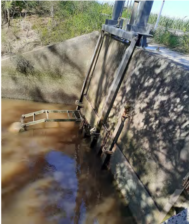
Figure 8-63: Example of a modified floodgate with a buoyancy gate and lifting device on the right bank floodgate (Floodgate ID F-2910-FB-0001)
