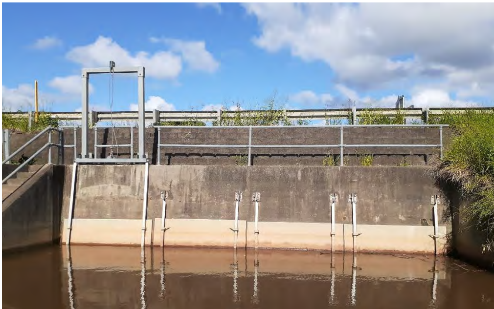
Figure 8-20: Floodgate ID F-2200-FB-0001 with vertical lifting mechanism on the right bank floodgate
