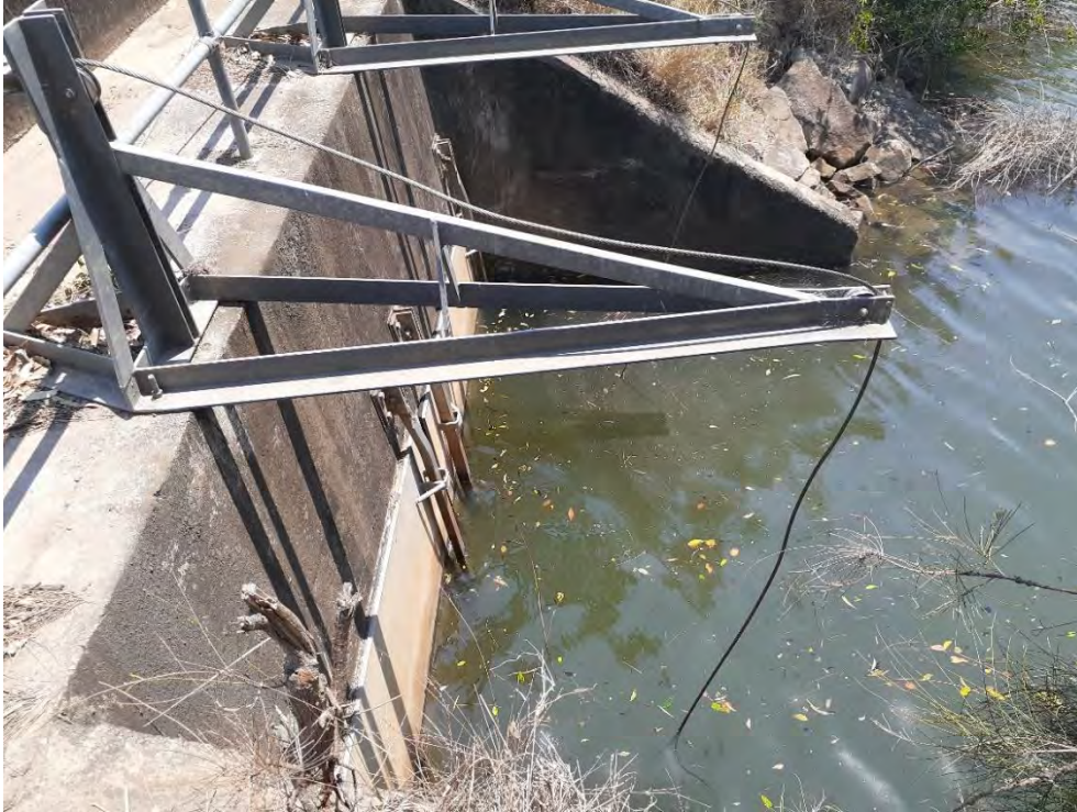
Figure 8-19: Floodgate ID F-2340-FB-0001 fitted with winch mechanism
