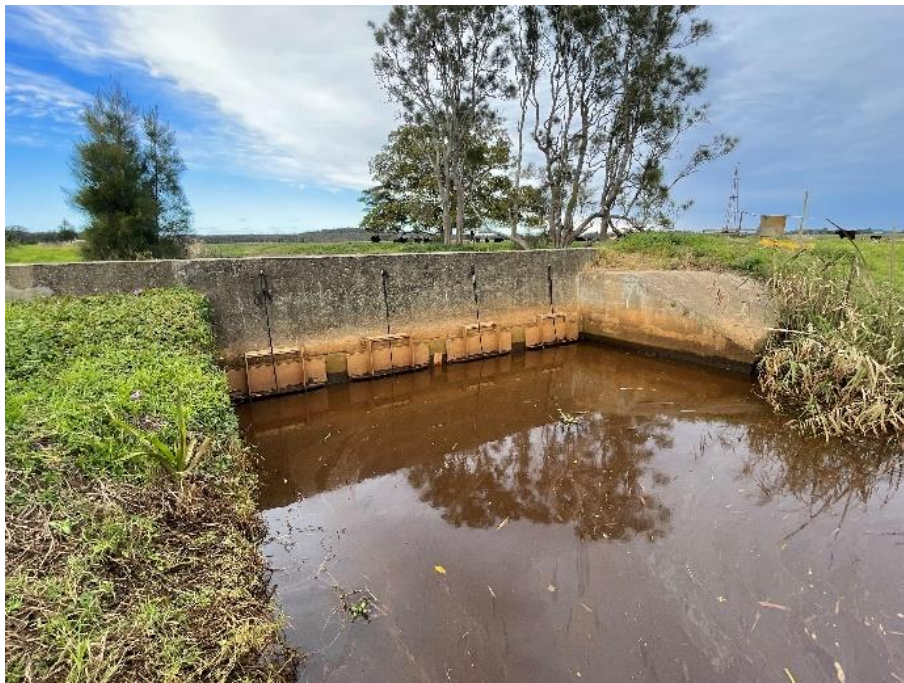
Figure 8-46: The Lock without auto-tidal floodgates (June, 2021) (Tucker and Rayner, 2021)
