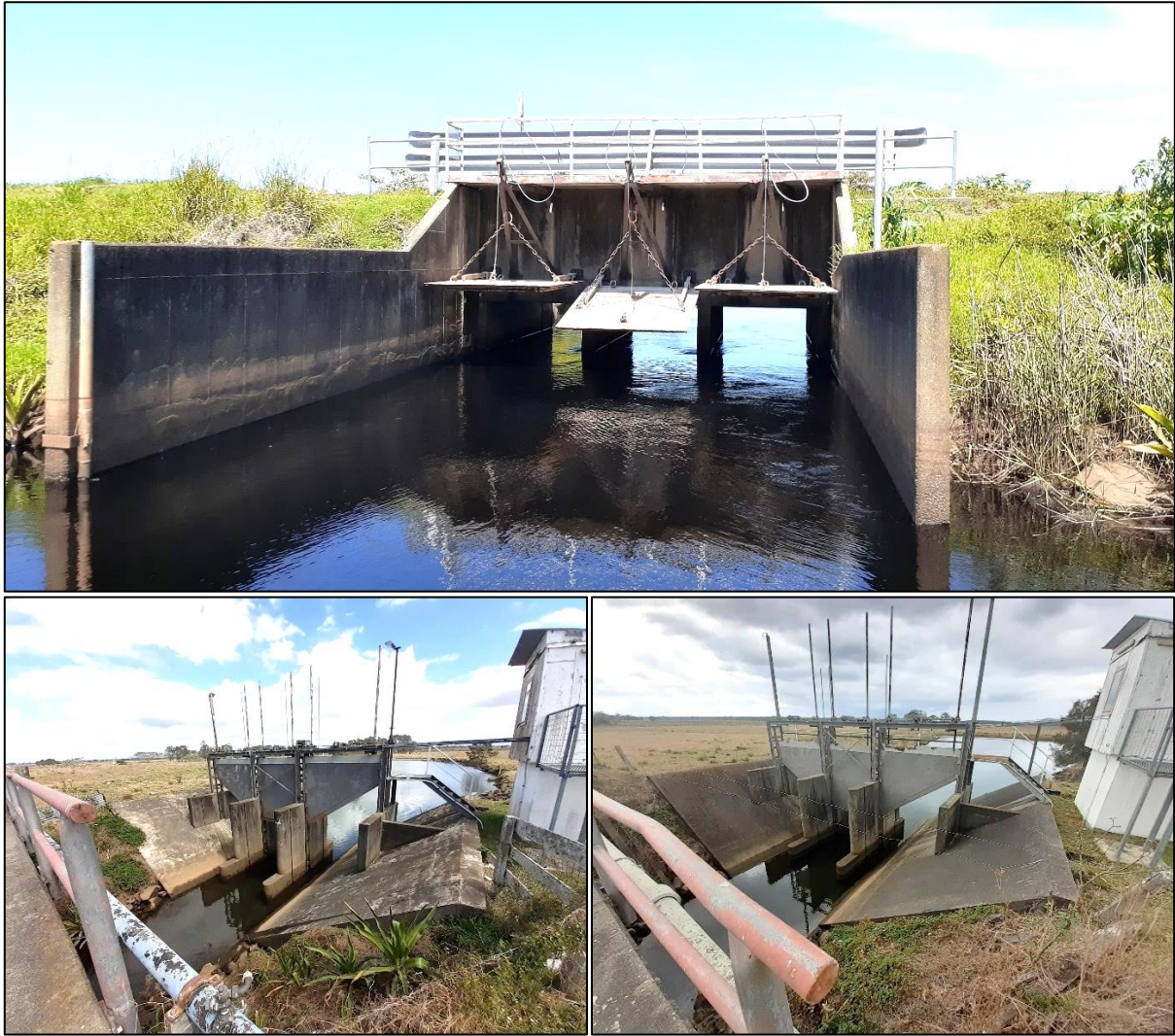
Figure 8-41: Major end of system flood control structures on Kinchela Creek including the Kinchela Creek headworks (024G1) (top), Kinchela Creek west floodway (025G1) (bottom left) and Kinchela Creek east floodway (026G1) (bottom right)
