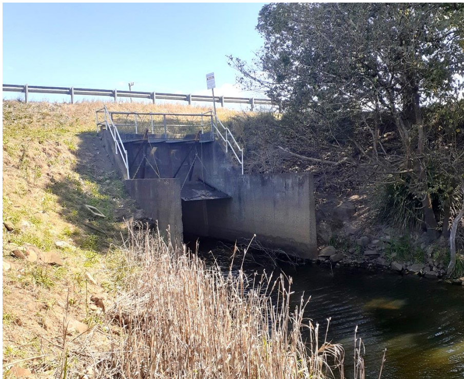
Figure 8-68: Euroka Creek floodgates (010G1) observed to be winched open during field investigations in September 2019
