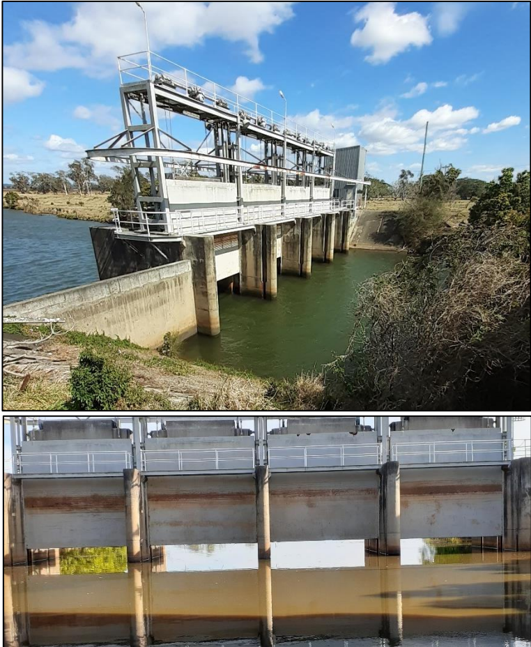
Figure 8-33: Belmore floodway structure (016G1) open when inspected in September 2019 (top) and March 2020 (bottom)
