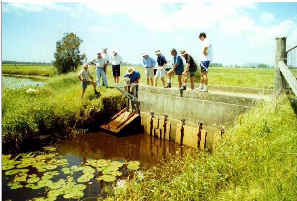
Figure 8-44: Lifting device installed on Wilsons Drain in 2000 (Tulau, 2011)
