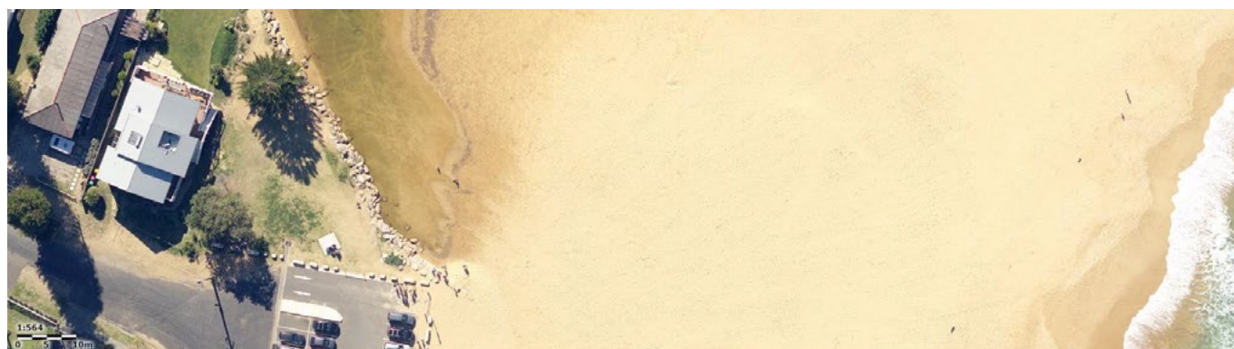
The rocks on the southern bank of the entrance channel were installed to limit the channel undermining the car park area
