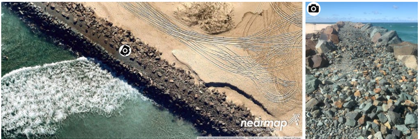
The rubble surface on the last 200 m of the northern breakwater of the Manning estuary creates a wildlife refuge area Credit: nearmap
