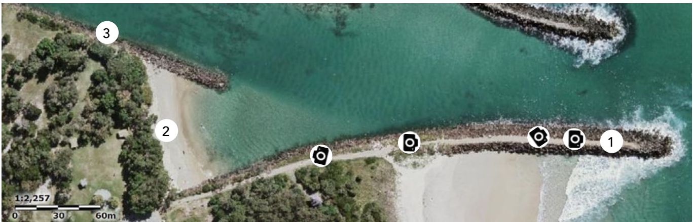
Brunswick River Breakwater: (1) the southern breakwater; (2) Torakina wave-trap beach; (3) part of the estuarine training wall Credit: Six Maps
