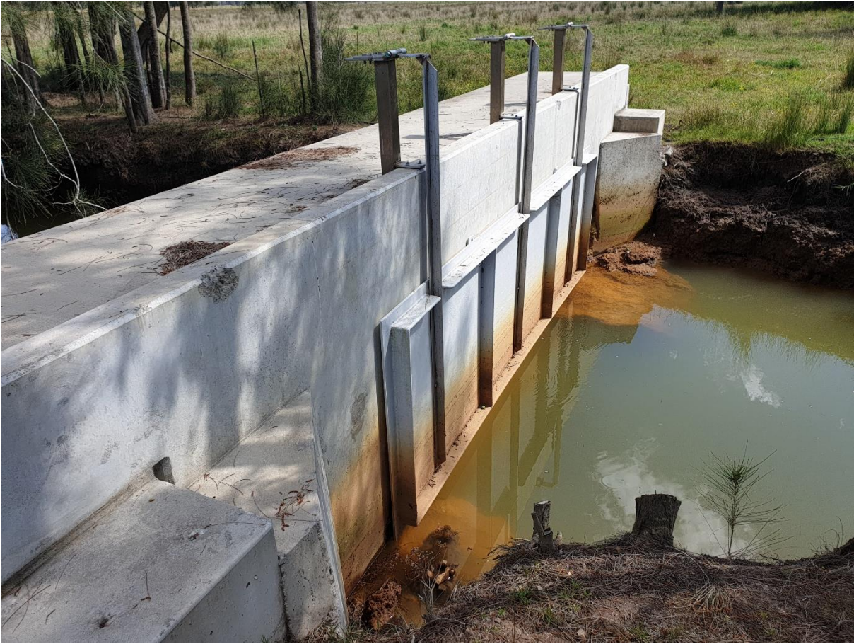
Figure 8-11: Floodgated weir at MANN031, invert 0.2 m AHD
