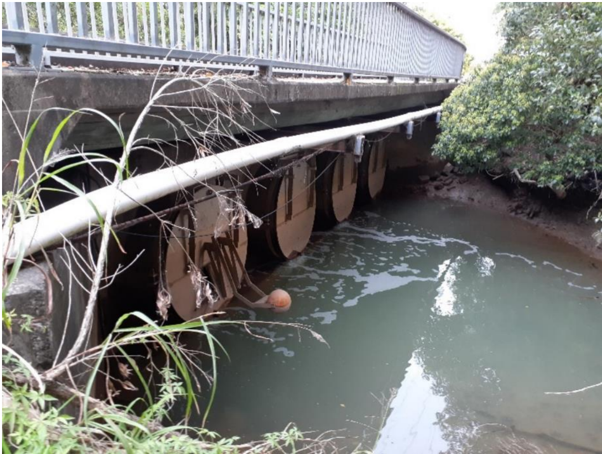
Figure 8-69: Buoyancy auto-tidal gate on floodgate 1280 at Montis Gully
