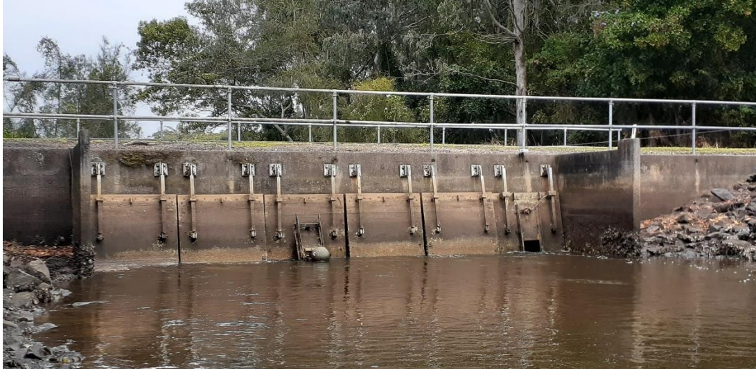
Figure 8-44: Floodgate ID 10 – at the end of the Keith Hall Drainage system (Photo: WRL, 2020)
