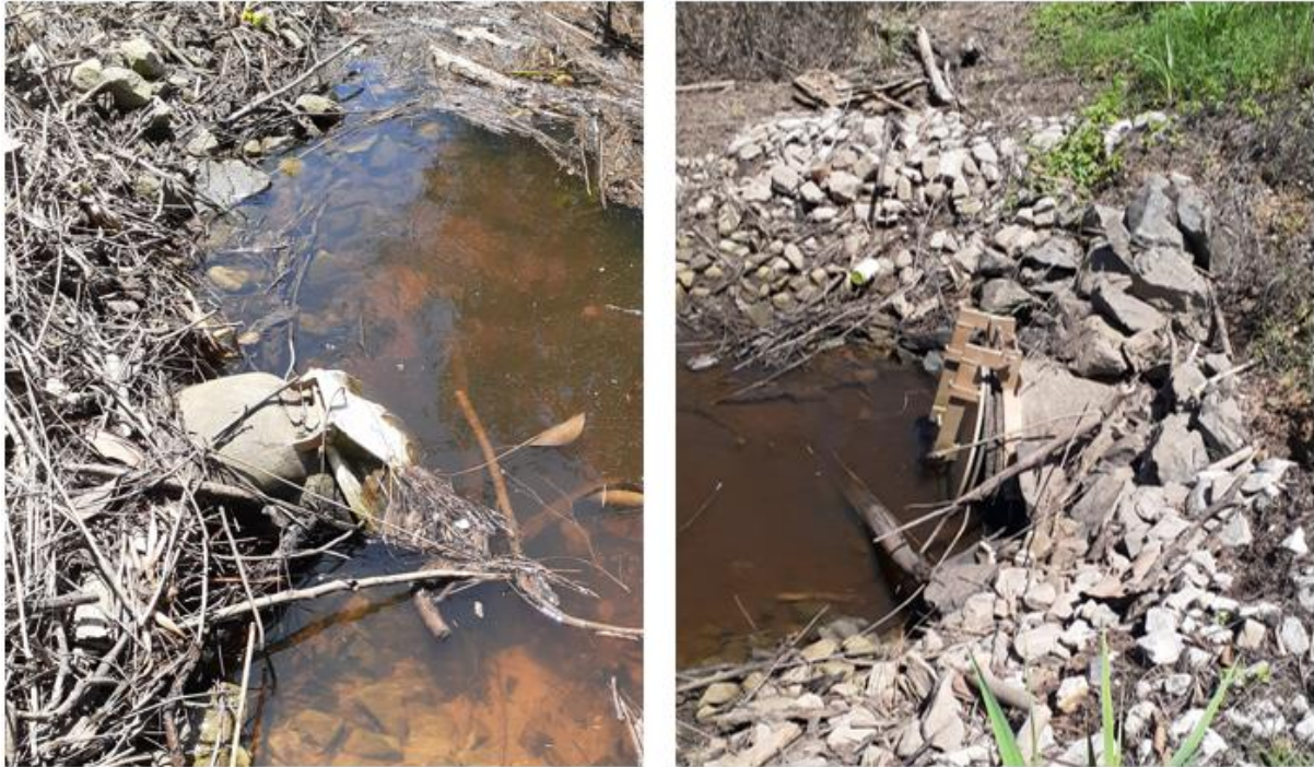
Figure 8-77: Example of floodgates wedged open in the Back Channel floodplain (floodgate ID: 4140 (left), 4100 (right))
