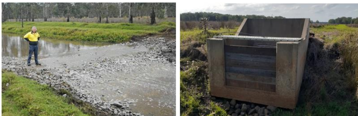
Figure 8-21: (left) Major rock weir at the downstream discharge point of Kookami Swamp (Source: Richmond River County Council (2014)) (right) drop board structure observed by WRL further upstream
